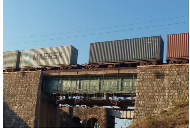
(b) After Strengthening
